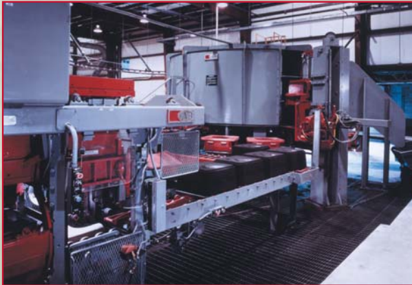
Automated foundry system to achieve good quality castings
